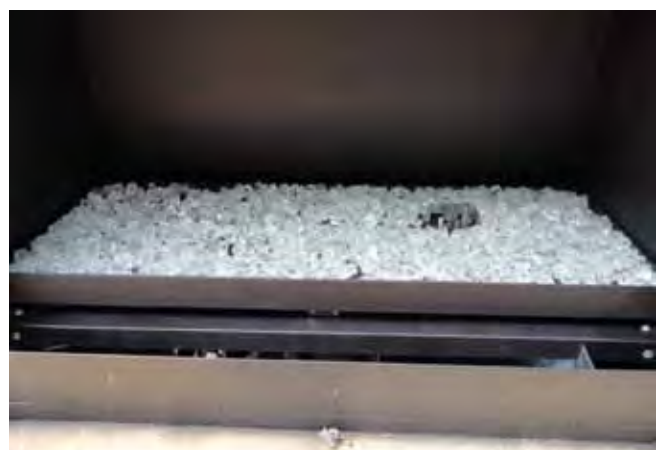
Figure 37. Firebox with media installed.
