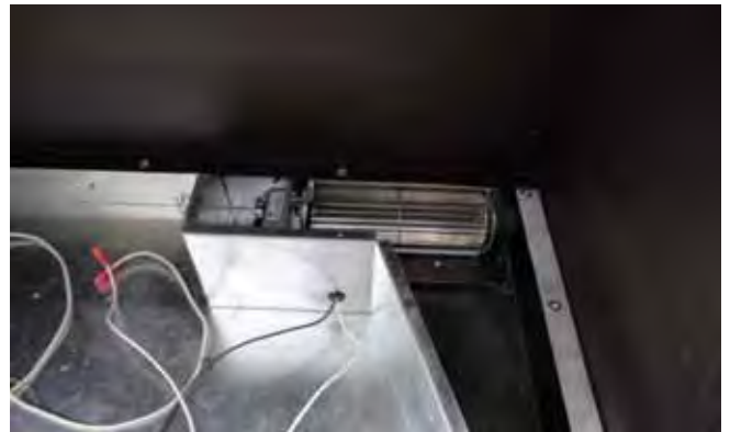
Figure 30. Location of blower.
